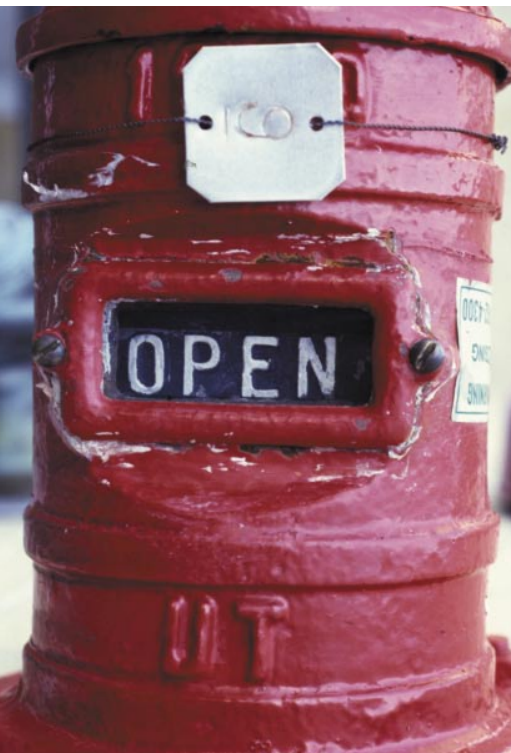
Lock all sprinkler valves open. A shut valve is the perfect catalyst for a successful arson strike. Sometimes arsonists shut valves, and then set the fire.
