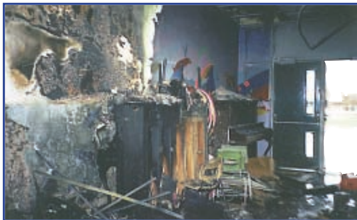
Fire damage to a school in November, 1998. Careless smoking is suspected.
